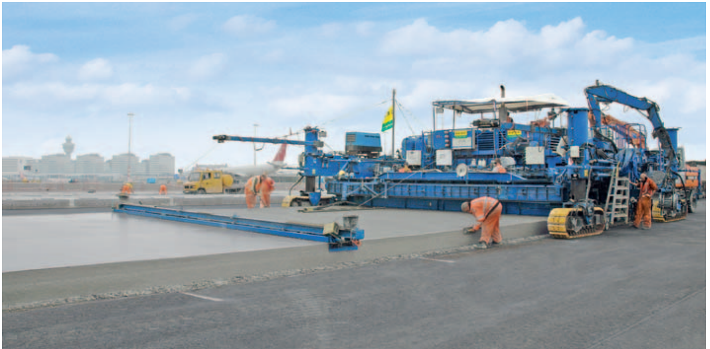
Wirtgen's slipform paver SP 1600 met the high quality demands at Amsterdam Airport, which specified a maximum tolerance of 5 mm over a length of 3 m in both longitudinal and transverse direction, with superior ease.
