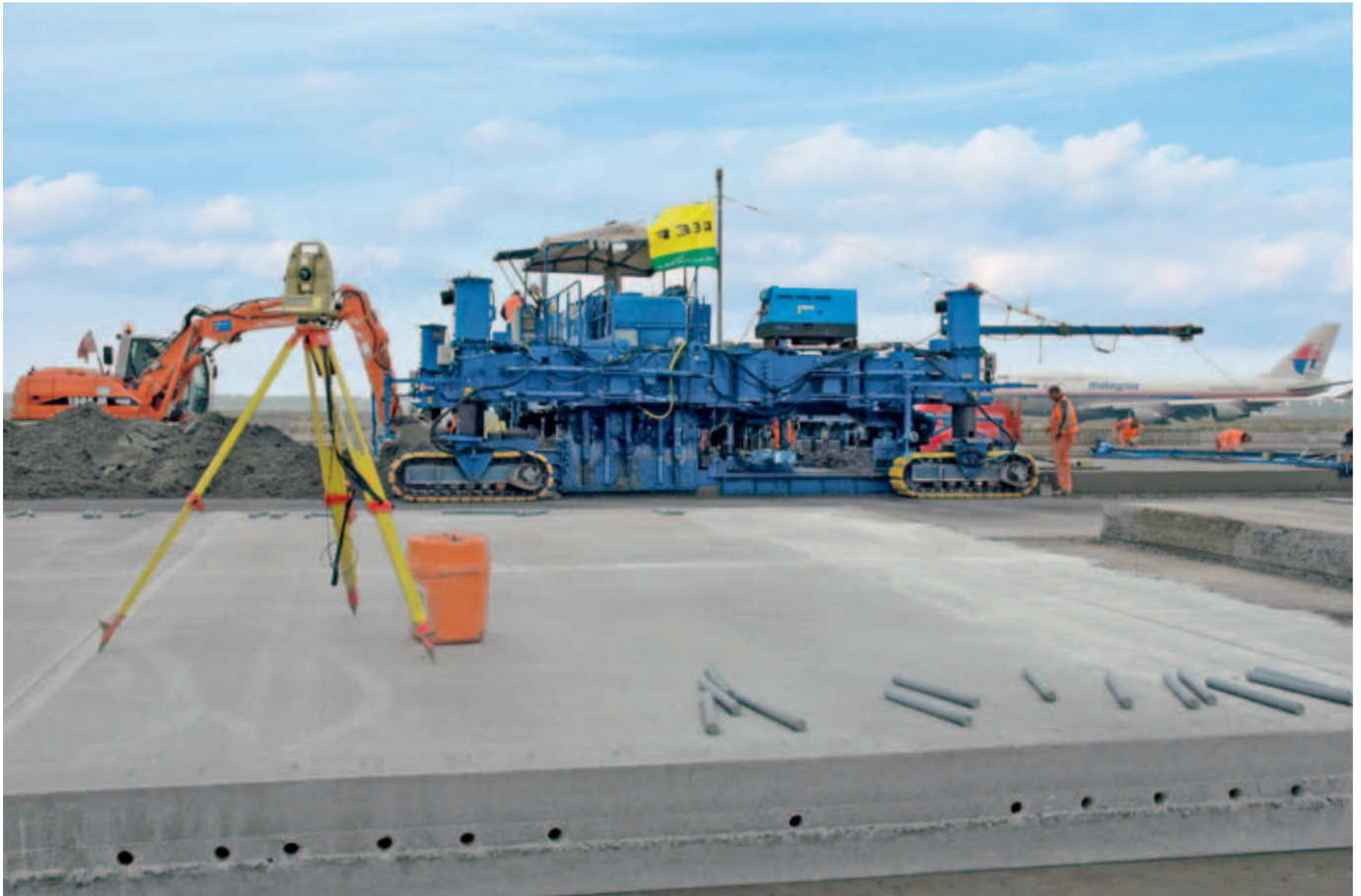
Modern concrete paving using Wirtgen's wireless control system instead of accident-prone and error-prone stringlines: The concrete cross-sections precisely matched the specified requirements of the digital terrain model.
