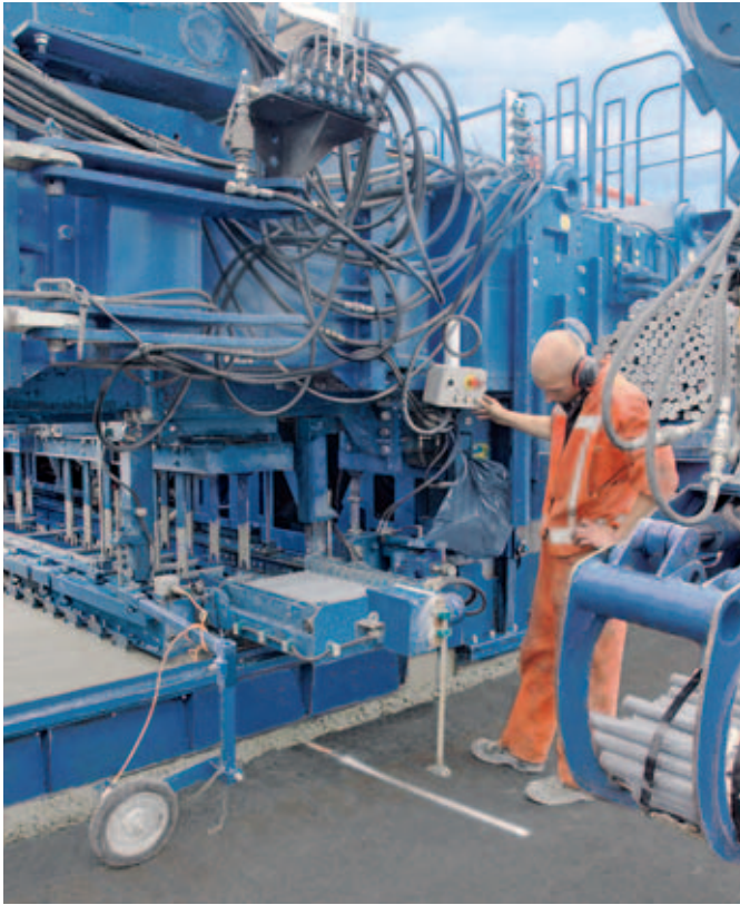
Loading the dowel bar inserter is semi-automatic, after which the dowel bars are inserted automatically at the push of a button.
