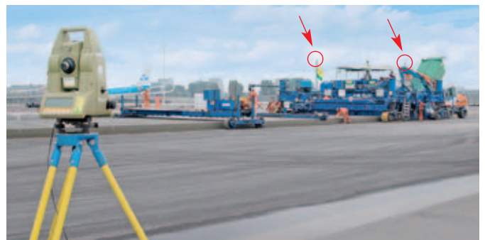
The total station is equipped with ATR (Type Leica TCA 1800), which enables it to automatically keep the prism on the paver in full sight.
