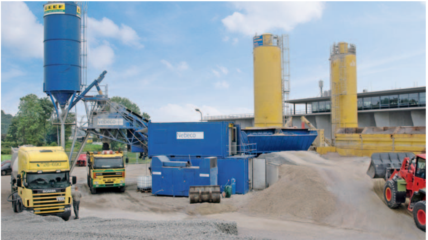
Two concrete mixing plants with hourly capacities of 200 and 50 cubic metres respectively processed granite gravel from Ireland and sand from the Dutch part of the North Sea, producing a total quantity of some 2,000 cubic metres of B55 grade concrete per day.
