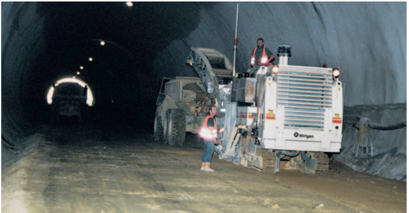
After blasting the surface was uneven and had to be cut up to 80 cm in depth. The 2100 SM was equipped with an integrated laser controlled levelling system and cut the surface precisely to the required level.
