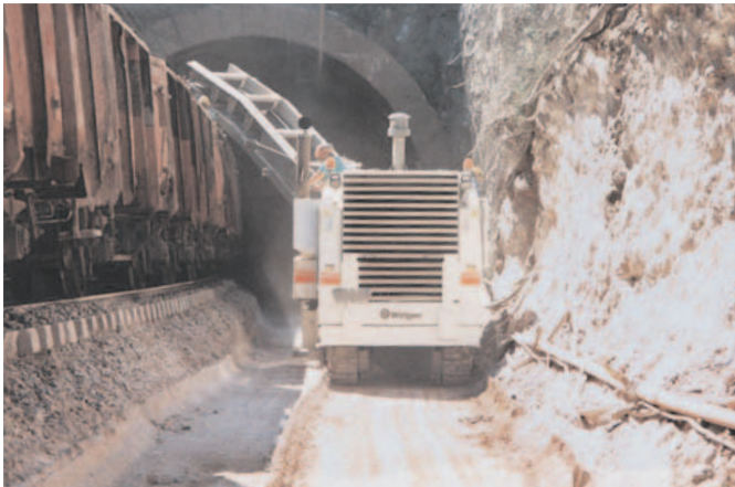
The 2100 SM was able to load the cut material directly onto train wagons travelling on the railway track.
