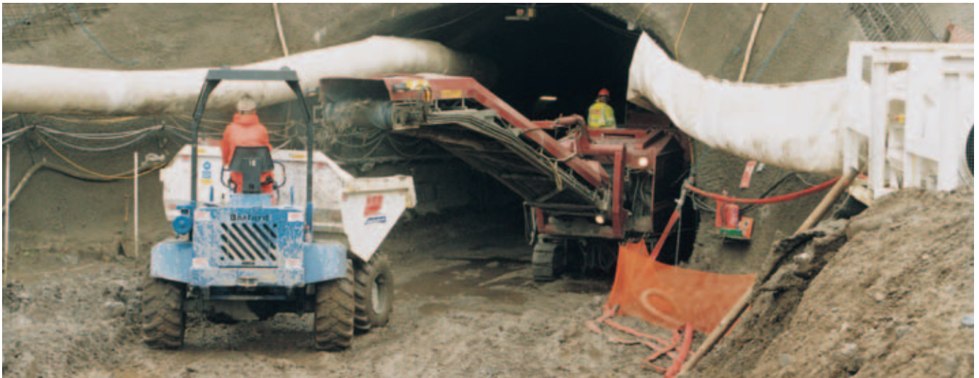
The 2100 SM cut series of stepped layers down to the final width of the tunnel floor. The result is a precise surface cut true to line and level.
