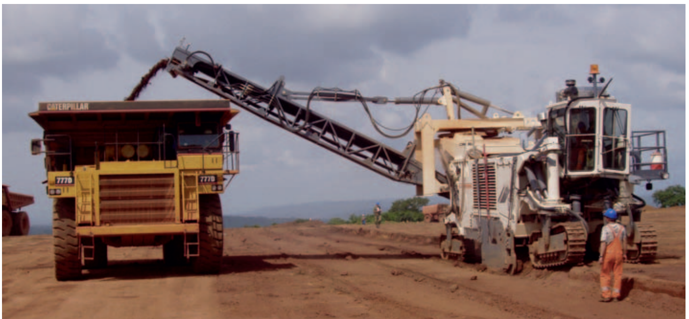
The direct loading of the cut material facilitates the operational processes in open-cast mining.
