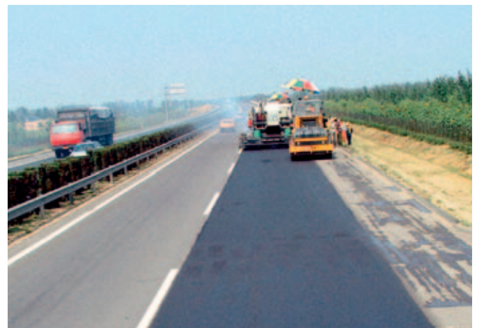
Showing the advantage of using hot in place recycling to recycle only the damaged slow lane.
