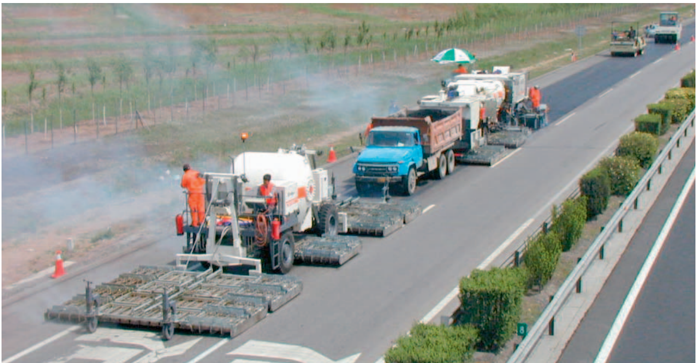
Wirtgen hot in place recycling on the Jing-Jin-Tang expressway between Beijing and Tianjin.
