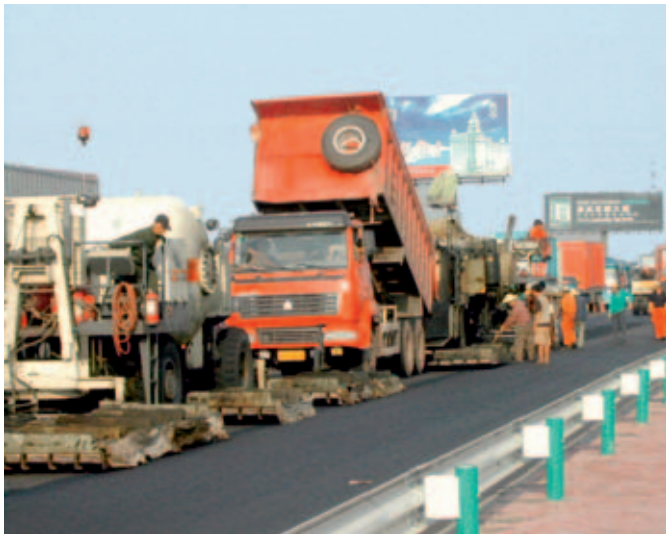
Hot in place recycling using the Wirtgen Remix-plus process on the Jing-Jin-Tang expressway.
