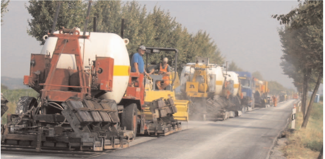
Fig. 4: Heating of the surface course. The first of the three panel heating machines is in the front area of the recycling set. The panel heating machines heat the old pavement to a temperature of 120 – 150°C.
