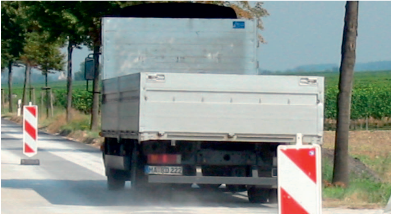
Fig. 15: When the asphalt layers have cooled down sufficiently, this section can then also be opened to traffic.
