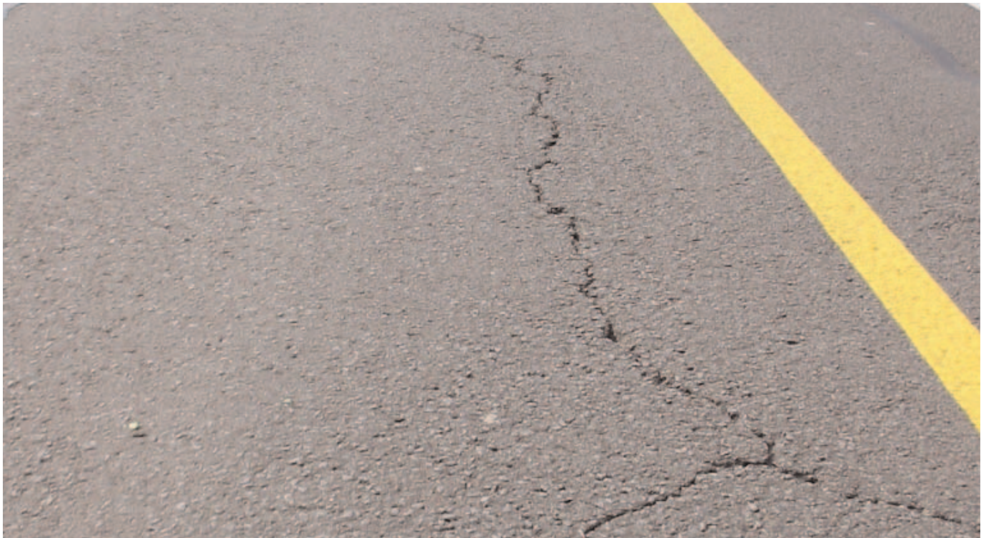
Fig. 2: Cracks in the surface course.
