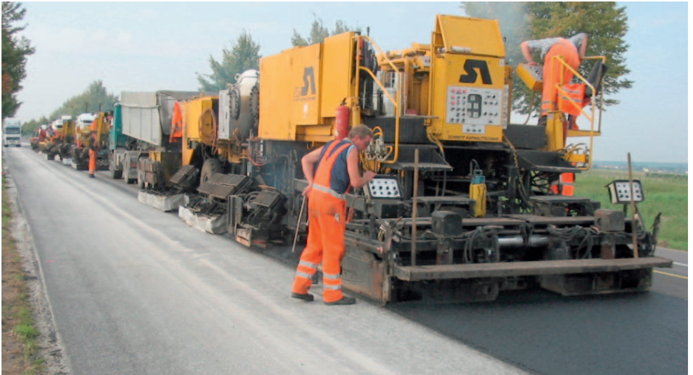
Fig. 11: "Hot-in-hot" placement: Virgin mix is laid on top of the remixed surface course.
