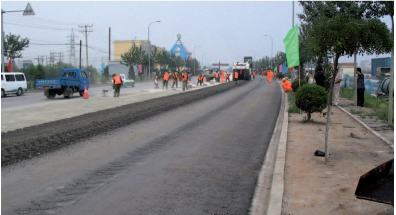
The cold recycling train with the WR 2500 S during the construction process.
