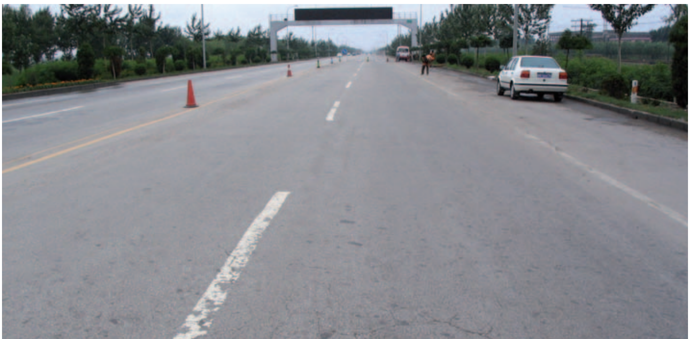
The condition of the old road before the rehabilitation with cold recycling.
