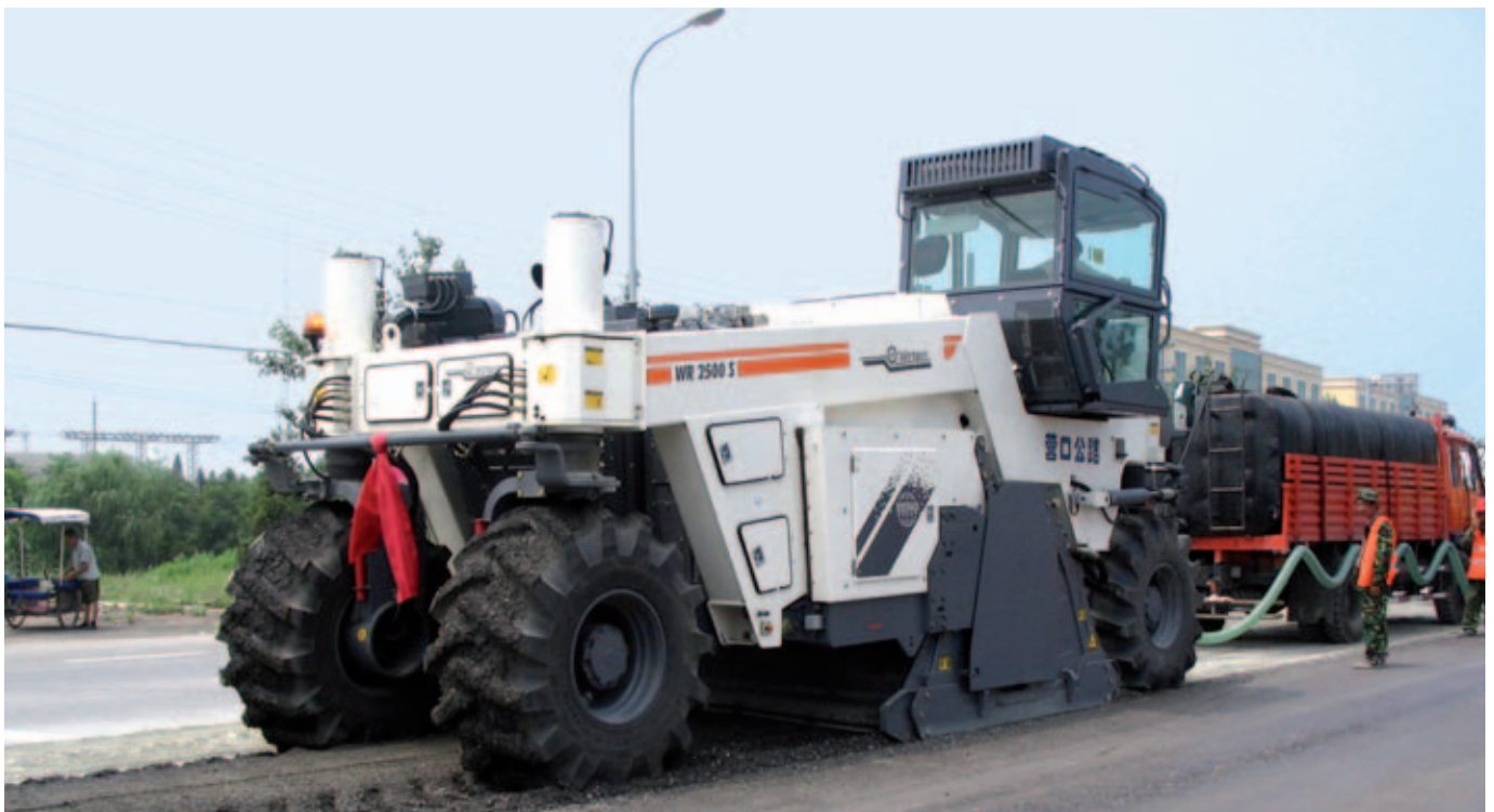
The all-wheel driven WR 2500 S is equipped with an injection system for both hydraulic and bituminous binding agents.
