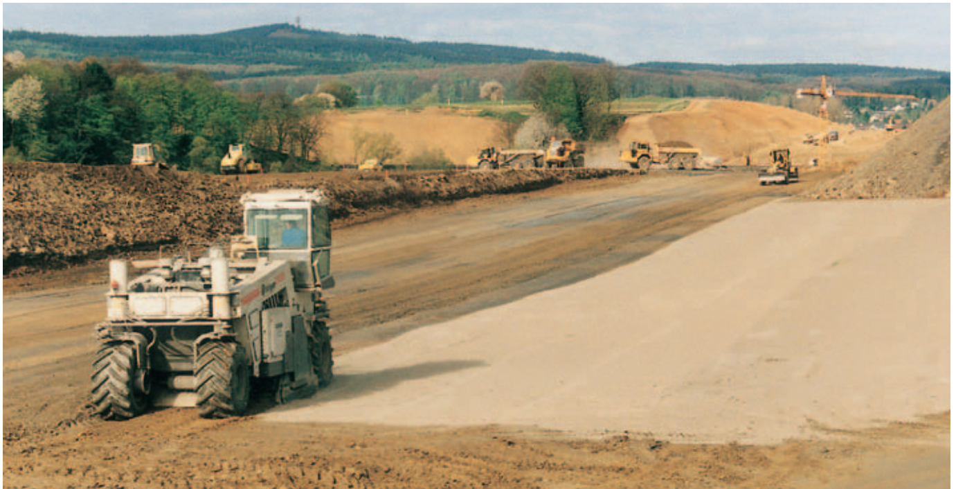
Overview on the construction site. In the foreground you can see the WR 2500 soil stabilizing with Terrafix.
