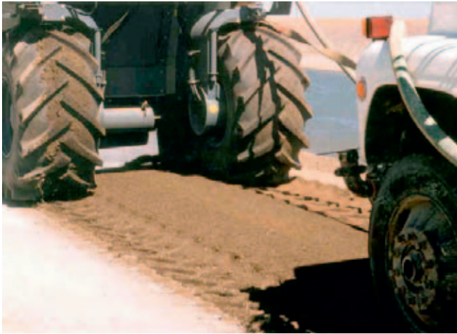
Road material after recycling with foamed bitumen (view between rear of WR 2500 and front of water cart).
