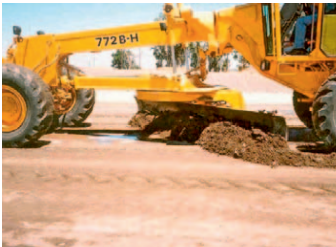
Following initial compaction with the steel drum compactor, the grader is used to cut the road to the required levels. The foam bitumen recycled material flows easily off the grader blade.
