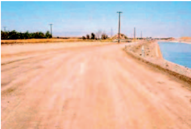
Final chipseal at junction with Creek Road, turn in area created during recycling process, 26 ft entrance, tapering to 14 ft road width.
