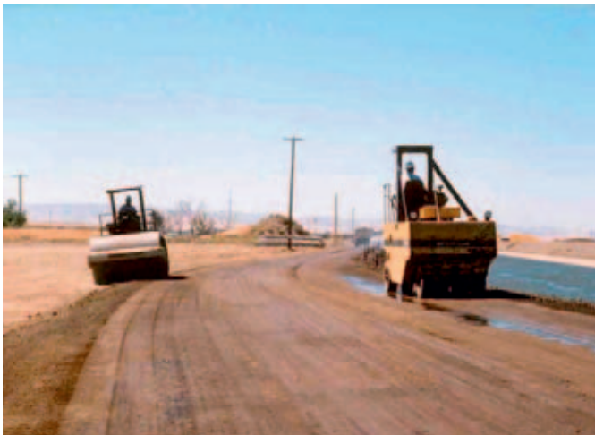
Required compaction achieved with 12 ton steel drum compactor. Surface finish compaction by means of multi tyred pneumatic compactor.
