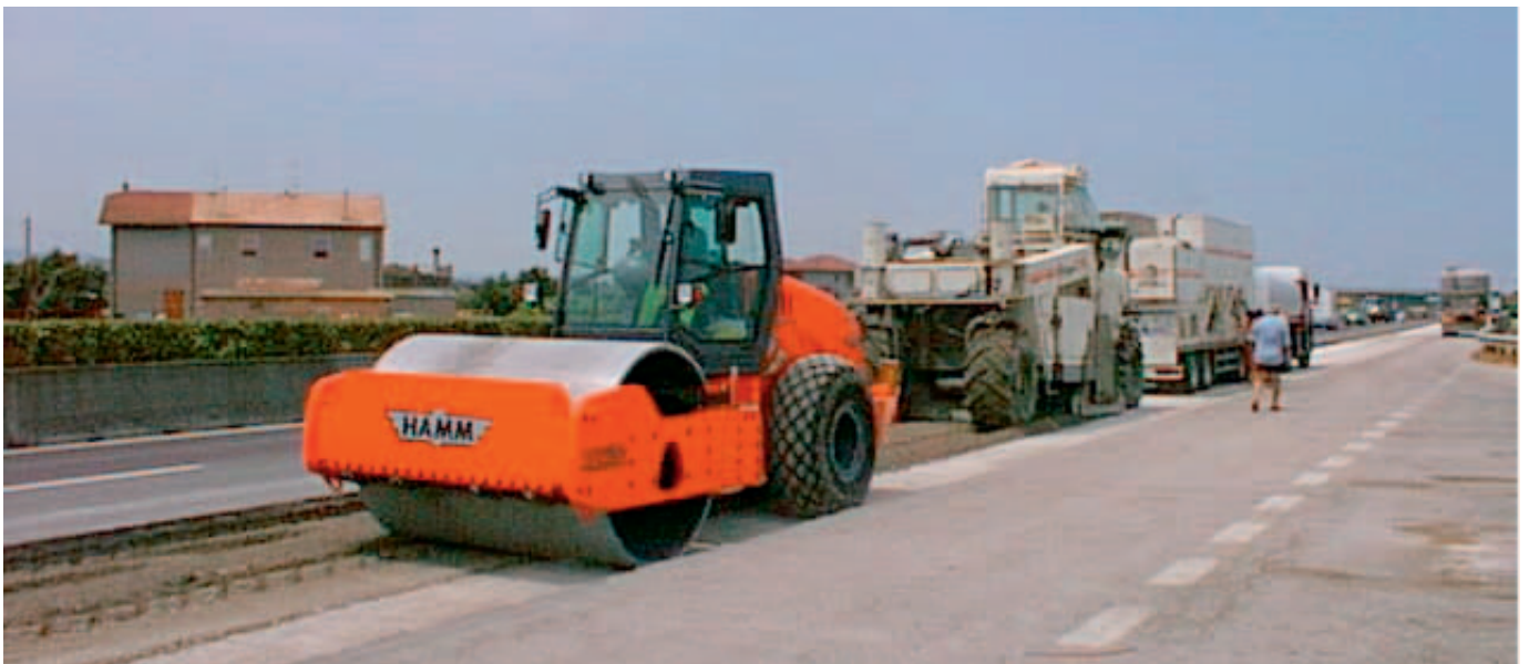
Fig. 8: Compaction taking place directly behind the recycling train using the Hamm 3520 HT.
