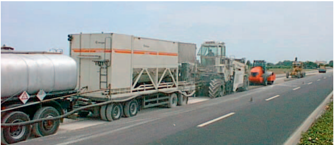
Fig. 10: The recycling train, consisting of a bitumen tanker, WM 1000 slurry mixer and WR 2500 recycler together with the compaction and finishing equipment processing the second pass.
