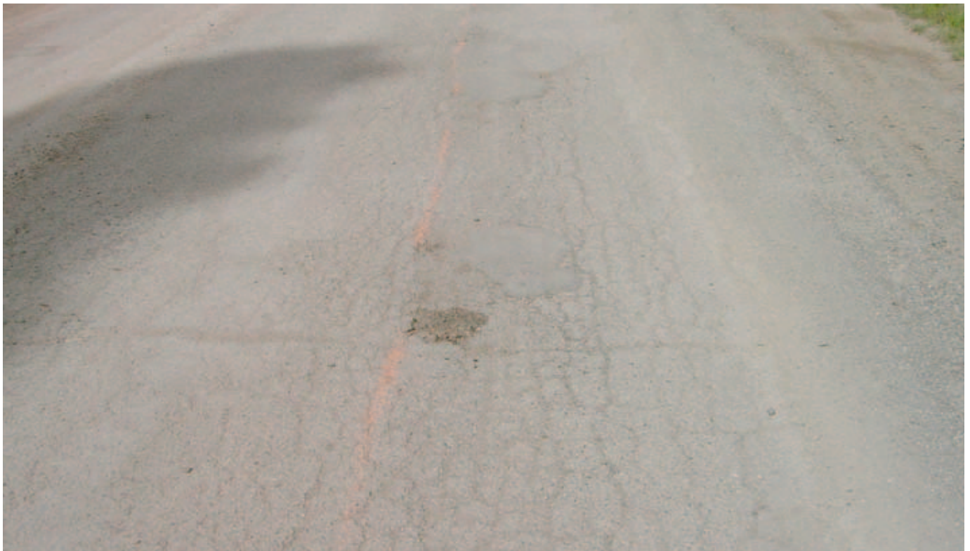
Typical view of pavement failure, extensive alligator cracking and associated base failure.
