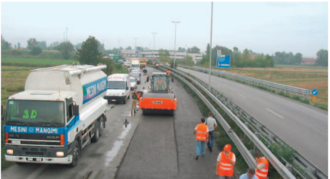
The compaction of the cold recycled base course is achieved by a Hamm 3520, which is a 20 ton single smooth drum vibratory roller, together with a pneumatic tyred roller.
