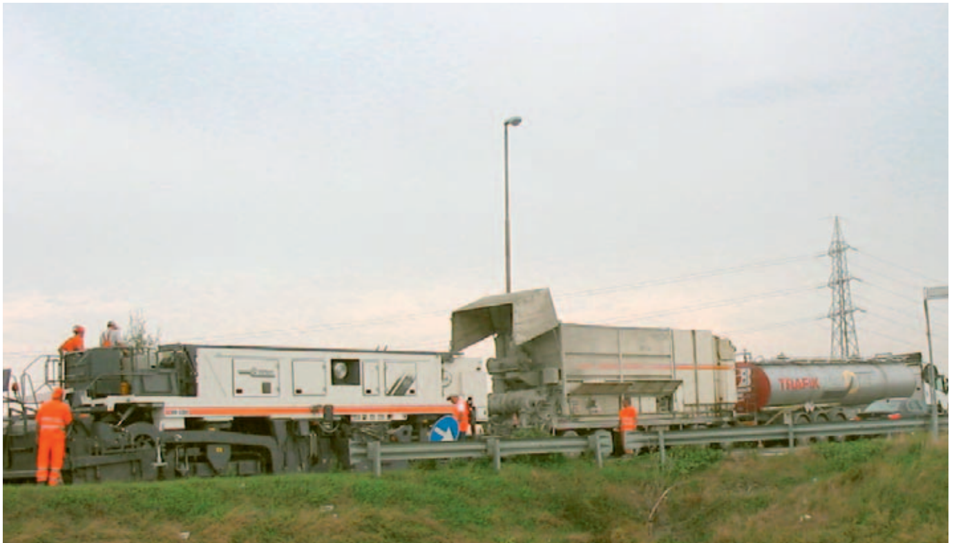
The recycling equipment coupled together by push bars to form one cold recycling unit consisting of the bitumen tanker in the front, the WM 1000 cement slurry mixer in the middle and the WR 4200 recycler at the rear, milling and finishing the cold recycled base course.
