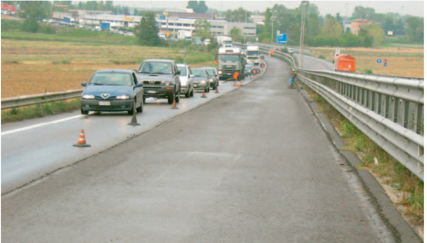
The finished cold recycled base course ready for short-term traffic and the asphalt wearing course.
