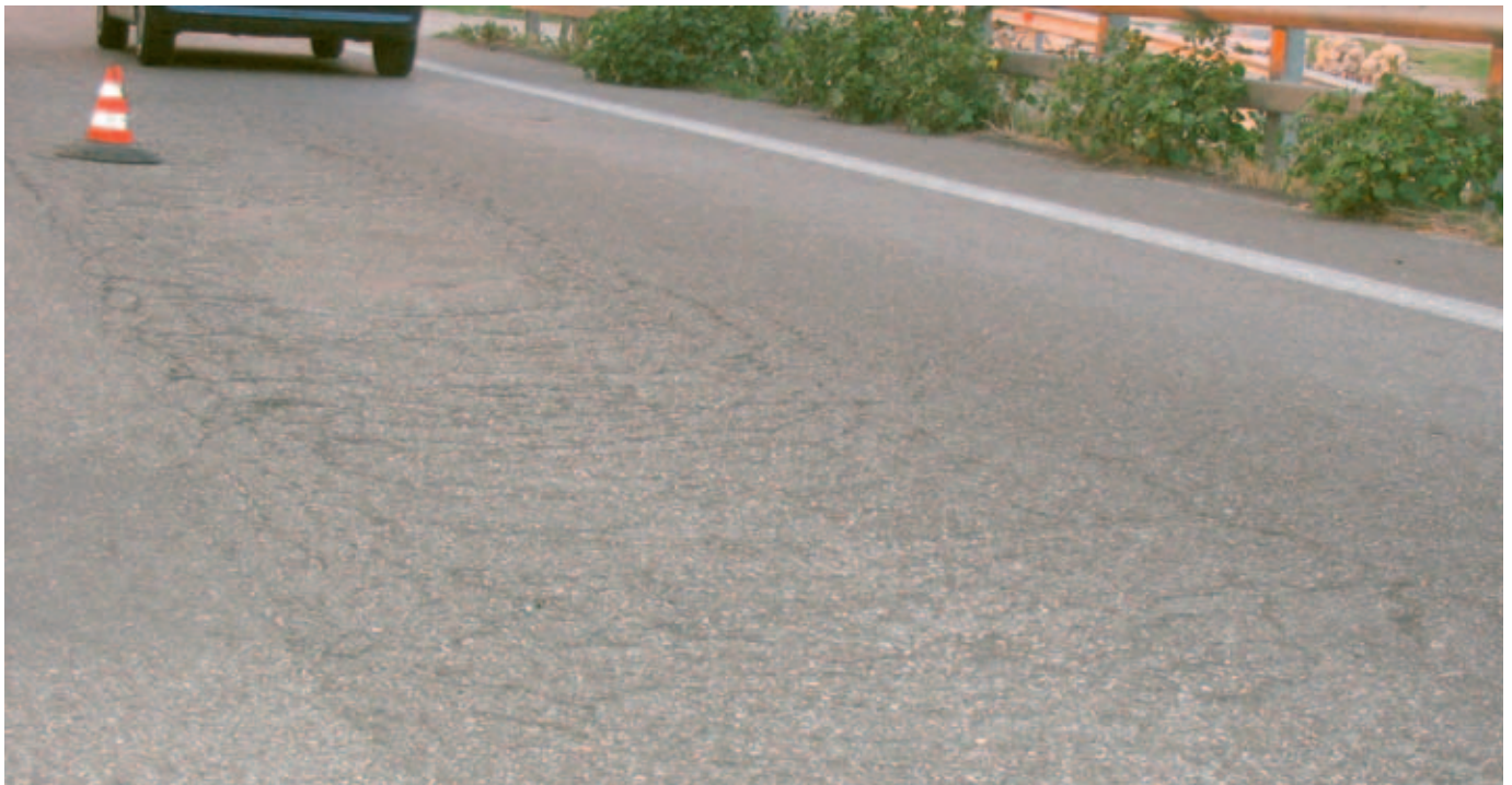
Road before rehabilitation showing severe deformation in the form of rutting and also crocodile cracking in places.
