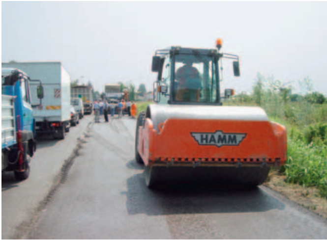
Finish compaction using Hamm 3520 single drum vibratory compactor, plus double steel drum vibratory compactor.
