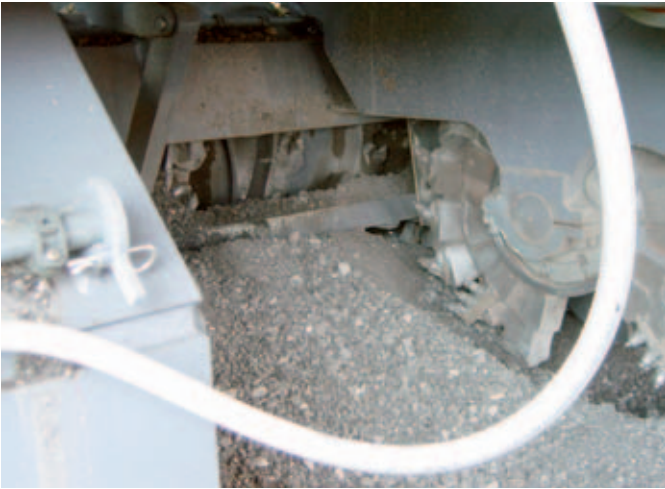
Hydraulically operated gradation beam fitted to central up cutter maintains particle sizing.
