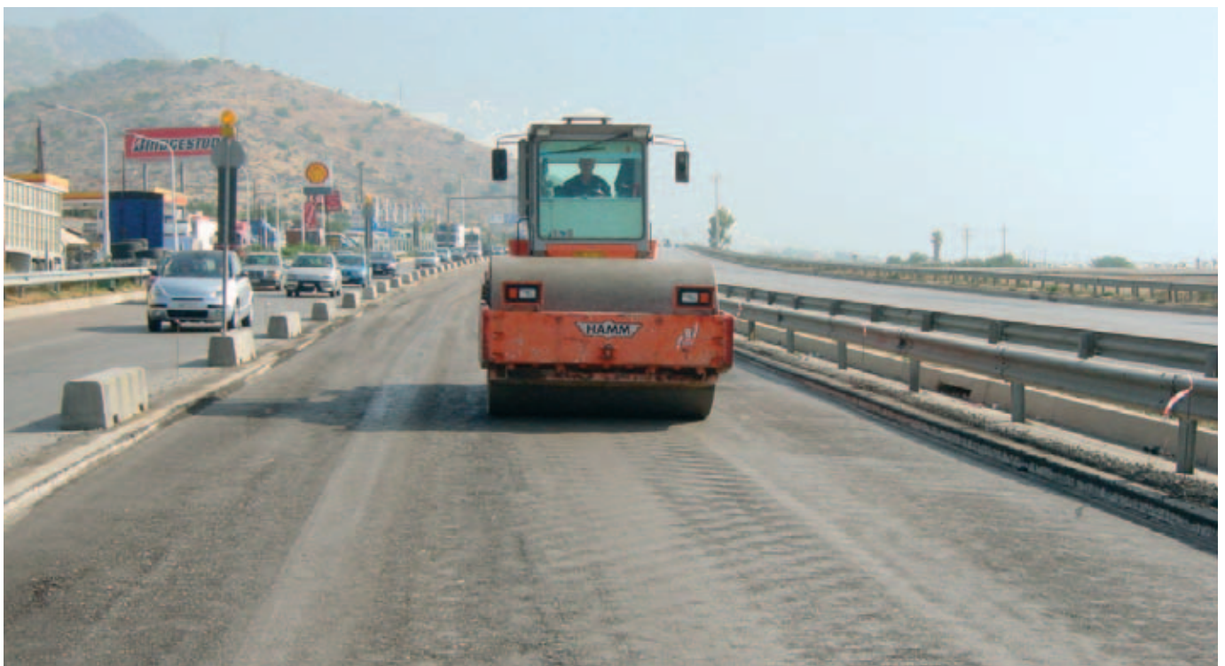
Finishing to achieve a tightly-knit surface using a pneumatic-tyred roller. Generous applications of water are applied whilst rolling, thereby generating a "slush" to close surface voids.
