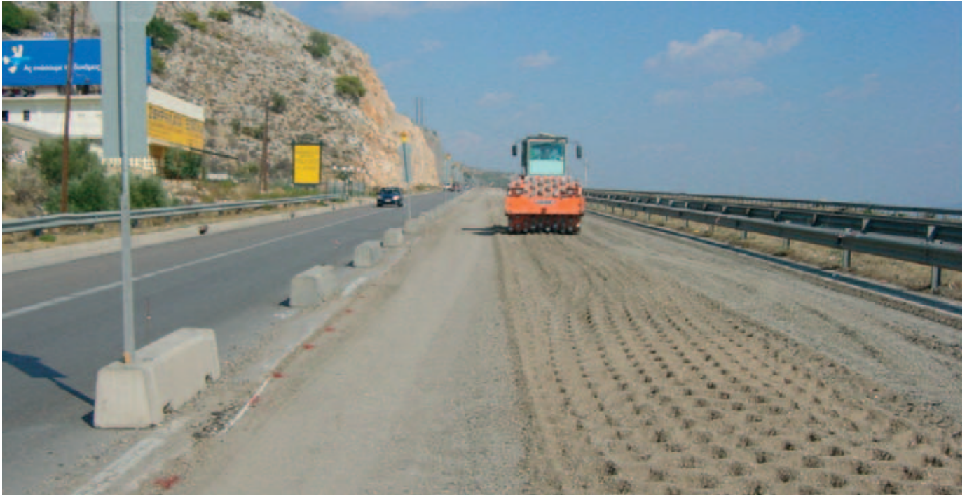
Primary compaction applied immediately behind the recycler by means of a 20-ton vibrating padfoot roller. This roller is fitted with a compactometer that monitors the degree of densification achieved in the recycled layer. Rolling continues until this meter indicates that the maximum density achievable has been obtained (normally between 9 and 15 uni-directional passes). The average density achieved is equivalent to 102 % of modified Proctor density.
