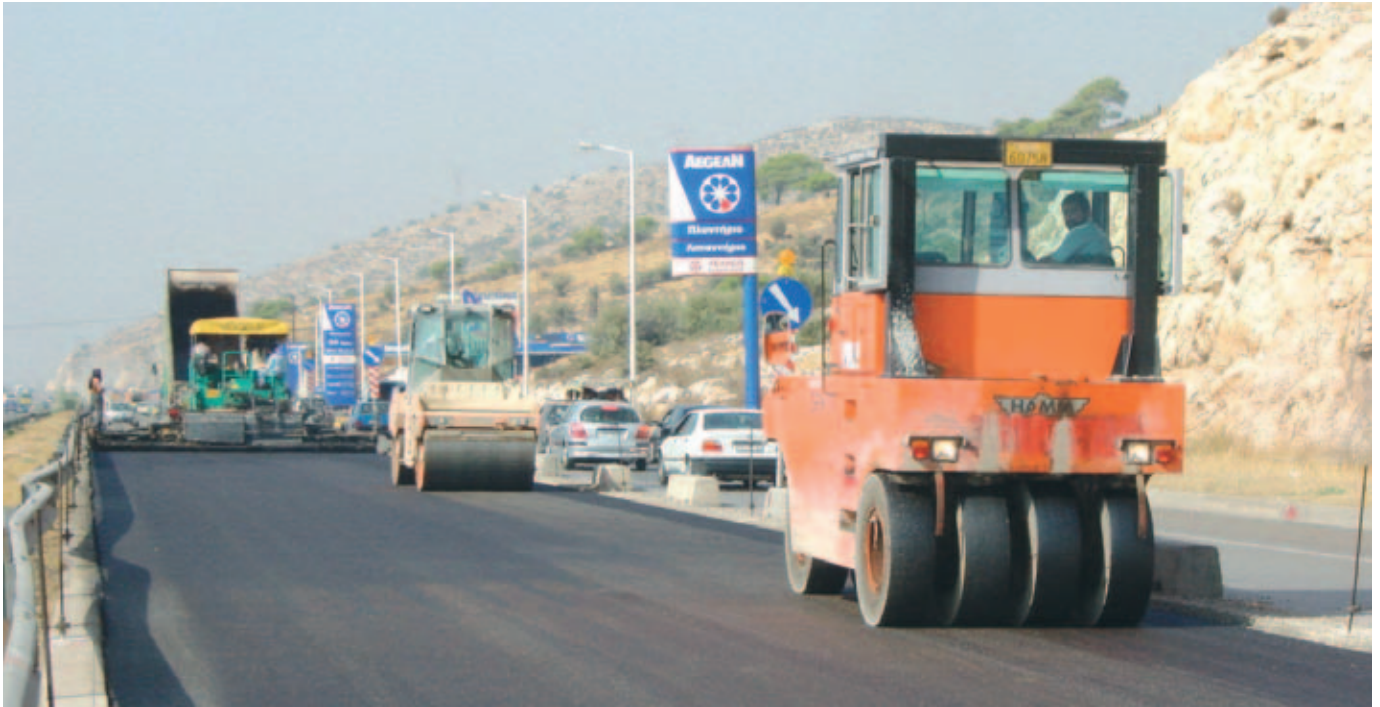
After compaction and applying temporary road markings, the traffic is moved onto the completed pavement.
