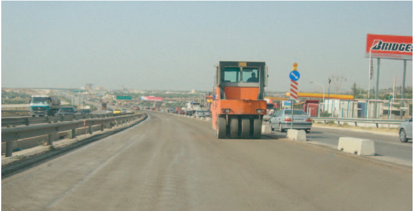
Compacting the upper portion of the layer disturbed by cutting levels using a smooth-drum vibrating roller. Water is sprayed on the surface prior to and during compaction, as demanded by ambient conditions.
