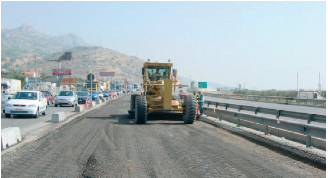
Cutting final surface levels by grader after the three adjacent cuts that have been recycled and compacted by padfoot rolling.
