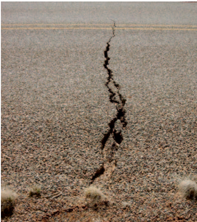
Full depth cracking through the asphalt pavement.
